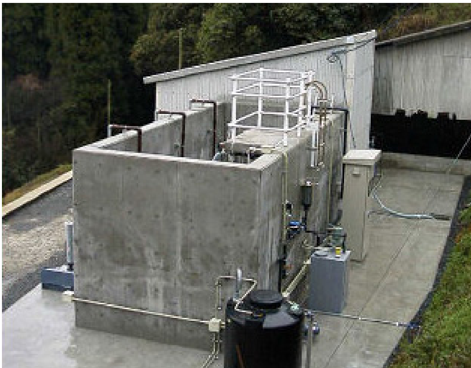
Overview of Treatment Plant
