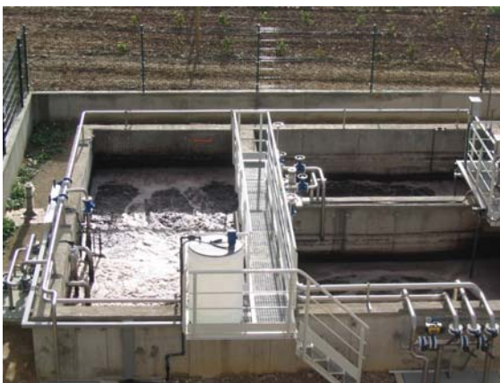
Fig 2.- Aerial view of the double biological reactor and the membrane chamber.
