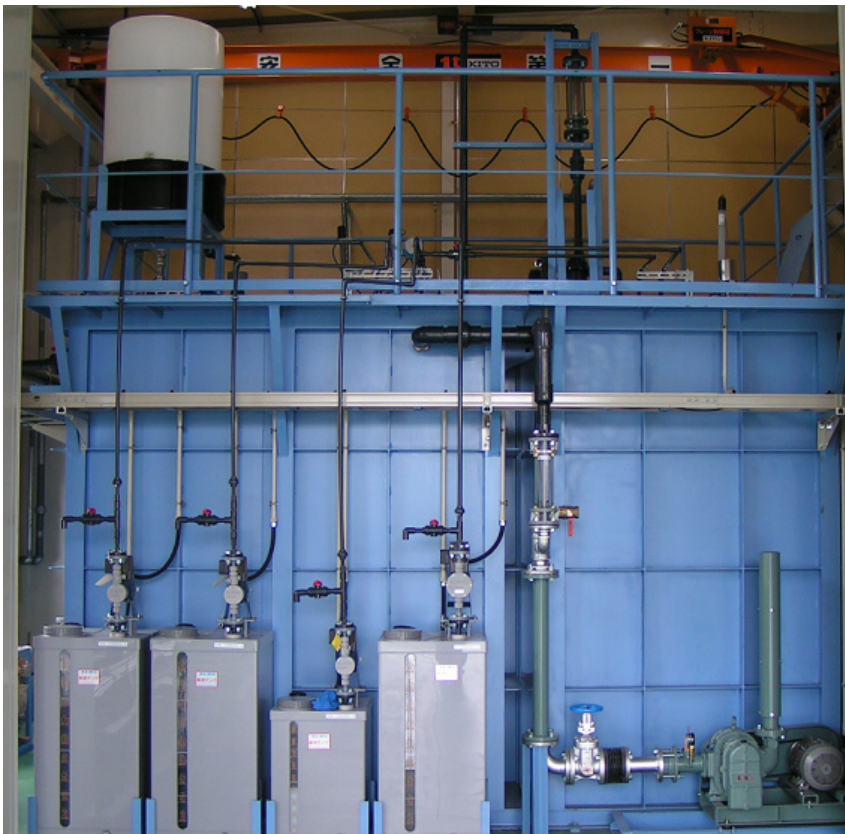
Overview of Treatment Plant
